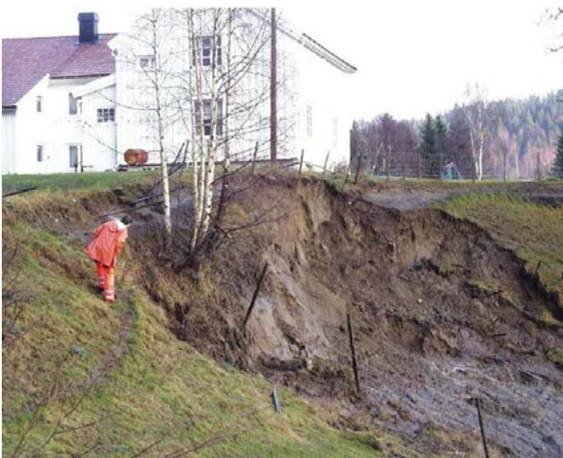
Figure 1. Landslide in sand and silt, Negarden Sander, Eidsvoll in Eastern Norway in the autumn of year 2000. Seepage of ground water visible from the foot of the landslide scarp.
