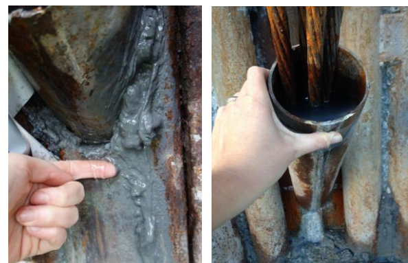
Figure 12. Example observed leakage in connection with installing tie-back anchors.
