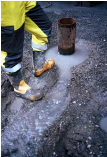
Figure 7. Observed leakage around drilled casing for steel core piles (Jernbaneverket, Jong-Asker).
