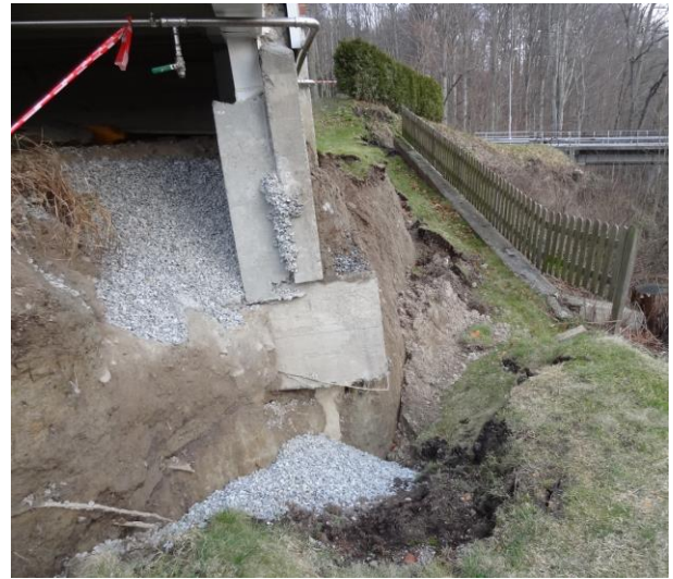
Figure 3 Backscarp of the landslide restricted by the pile foundation. Concrete pile supporting the corner foundation visible.
