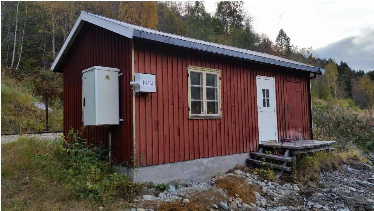
Figure 7: The cabinet containing the gateway is installed on the wall of a building by the entrance to "Vendetunellen". The gateway is the only system component requiring grid power, and this location was chosen as it is the only Railway owned installation within radio distance from the test site, with available power. The larger cabinet on the opposite wall is a GSM-R installation, enabling possible future integration of the system with existing railway telecommunication.
