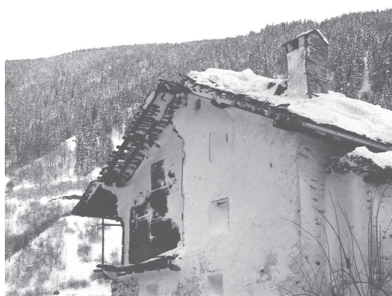
Figure 1: Signs of "air blast" impacts: top) snow deposits and damage caused by the 'skredvind' of the powder snow avalanche from Stortuva, Mosjøen, Norway, on 29.02.1996 (photo NGI); bottom) building damage caused by the Meira powder snow avalanche, Arviggio, Switzerland, on 12.01.1977 (photo Canton police, Grisons)
