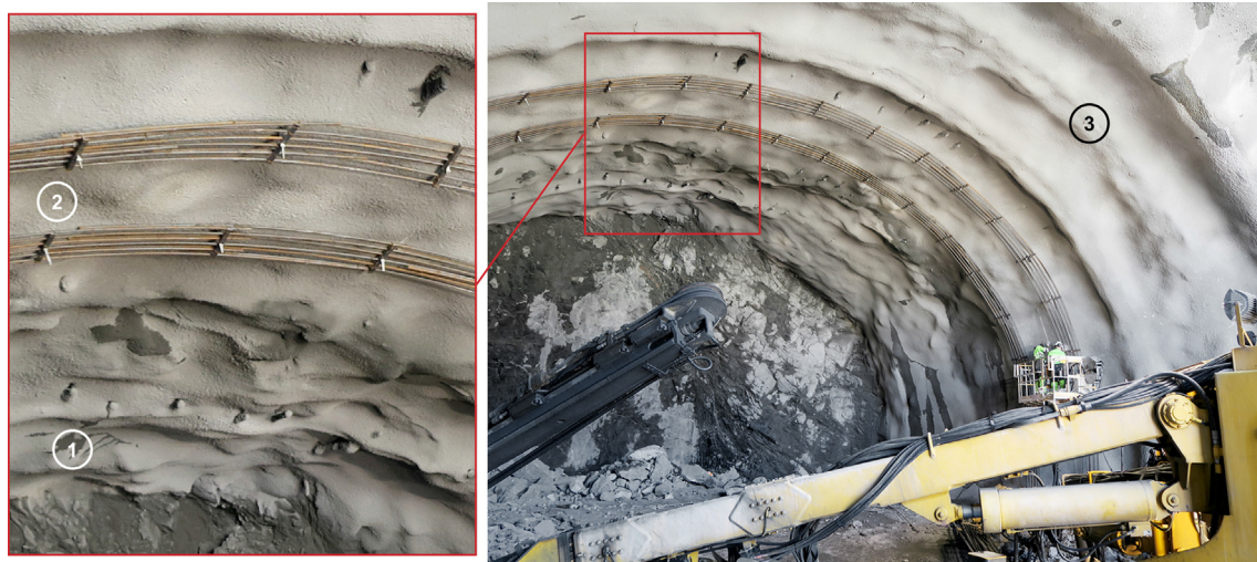
Fig. 1. Mounting of rebars for two RRS for permanent support (2). Further toward the face two (1) blast rounds are temporarily supported with spiling bolts held in place by steel straps and radial rock bolts. Finished RRS can be seen to the right (3).
