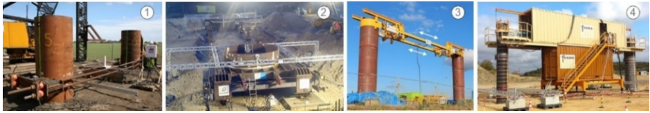
Figure 17. Large scale lateral pile load tests performed for investigation of P-Y response for monopiles: (1) Rødbyhavn (Denmark) - hard clay and driving shoes, performed by NGL/Bilfinger for Equinor (2014); (2) Cuxhaven (Germany) - dense sand and vibrated piles, performed by Bilfinger for RWEinnogy (2014); (3) PISA project, Cowden (UK) - stiff clay and Dunkirk (France) - dense sand, performed by ESG for Carbon trust consortium (2014-15); (4) Gouvieux (North France) - Sandstone, performed by Fugro for EMF (2016).
