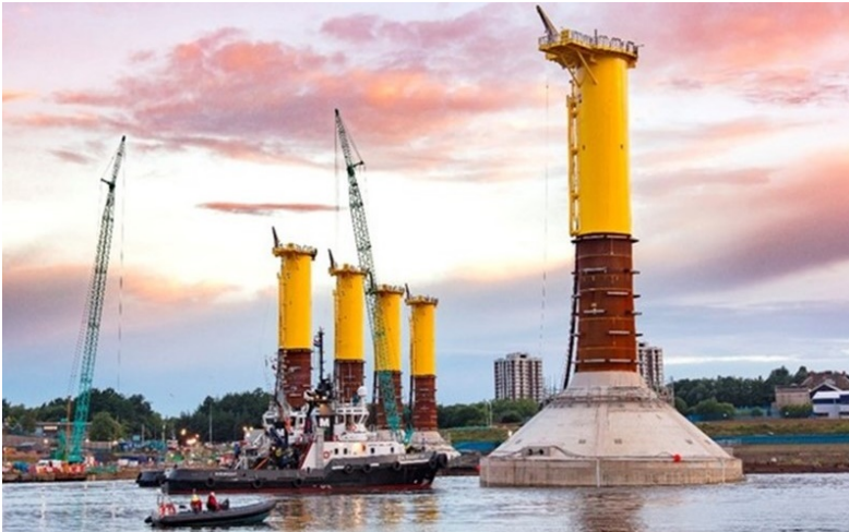
Figure 31. Tow-out of Gravity base foundations constructed by BAM for Blyth offshore windfarm.
