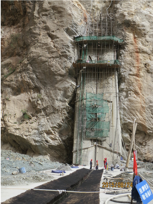
Fig. 2. View of the top of the foundation plinth and the plinth along the left abutment.
