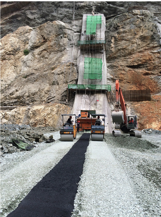
Fig. 12. View of the weak rock foundation along the right abutment at about half height.
