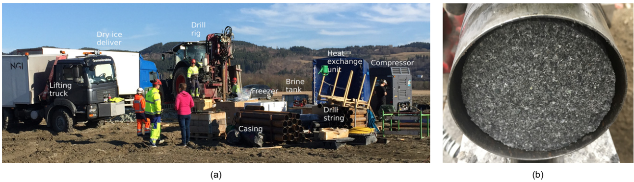
Fig. 3. Ground freezing technique used for field sampling: (a) overview of the installations needed at the site; (b) frozen Øysand sample obtained with this method
