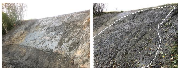
Figure 11. Man-made slope in Øysand site before (left) and after failure (right, April 2020)
