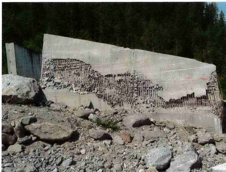
Figure 3.2: Deflector wall destroyed by the large Taconnaz avalanche in April 2006. The sensor was torn off before data could be transmitted to the logger.
