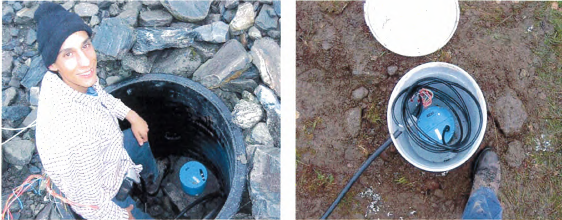
Figure 3.1.7 Detail of the installation of the 3-component LE-3D/5s Lennartz Geophones belonging to the University of Barcelona.
