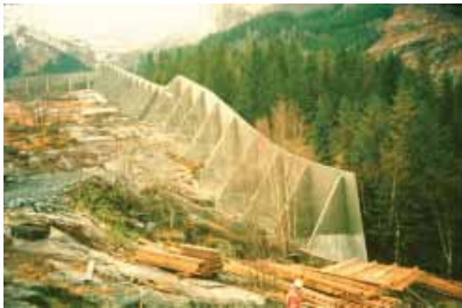
Figure 15.10: A concrete diverting dam at Odda, Norway (height 8 m, length 200 m) (photo: Karstein Lied).
