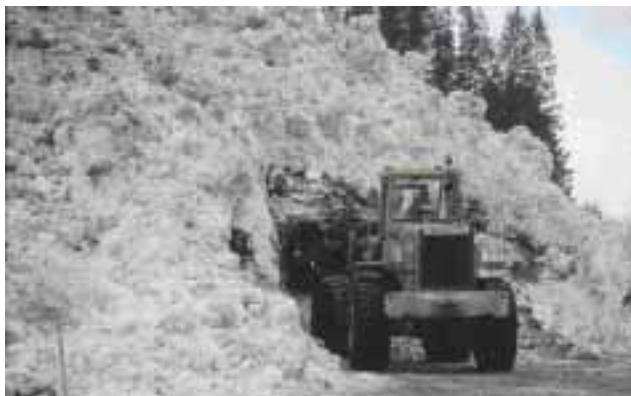
Figure 8.5: Large amounts of wet snow may pile up in flat areas when the front stops and additional volume from the tail of the avalanche accumulates on top of the snow that has come to rest (photo: NGI).
