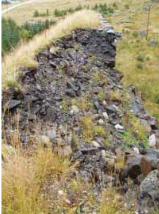
Figure 15.2: Failure in an avalanche retaining dam. The dam height is 8 m. (Photo: Karstein Lied.)
