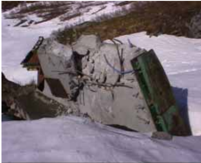
Figure 13.1: Damage caused by an impact of solid debris at the NGI test site Ryggfonn (photo: NGI; Avalanche event 20000217 13:55).
