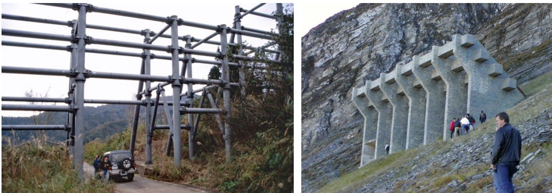
Figure 7. Semi-permeable structures for braking fast, large avalanches. Left: Steel structure near Maseguchi, Nagaoka Prefecture, Japan against powder-snow avalanches. Right: Large concrete structure in Austria. Images courtesy S. Margreth, SLF Davos.
