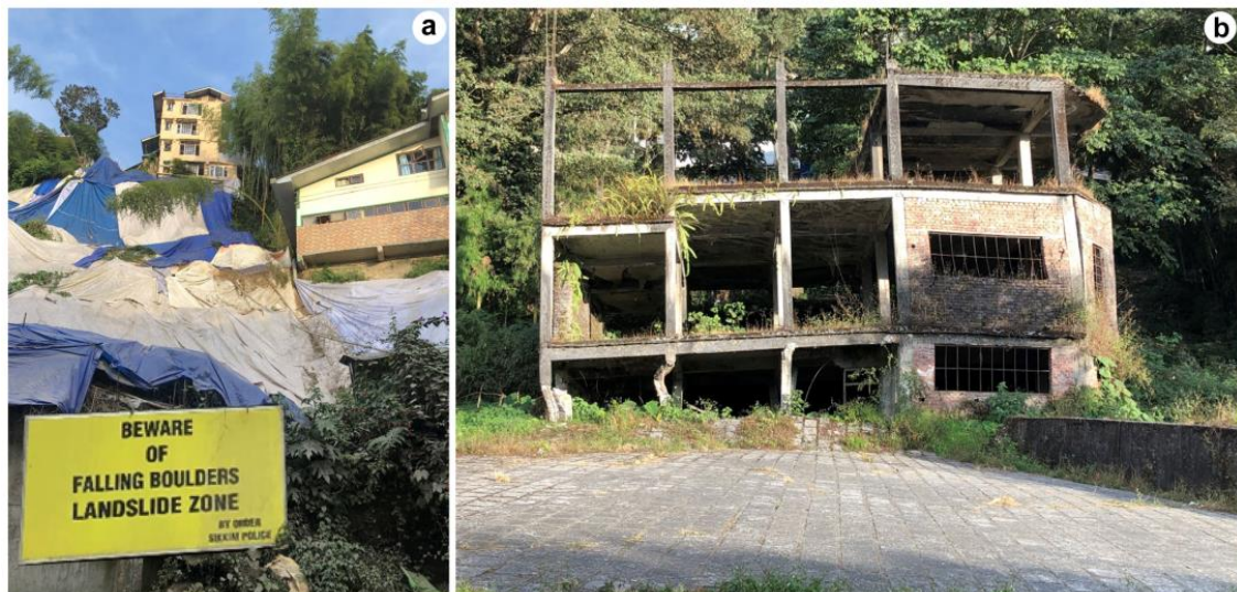
Figure 7. (a) Collapse of a residential building in Sichey where the area is covered with plastic sheets to avoid seepage of water from precipitation. (b) Abandoned construction of a Tibetan school in lower Sichey due to differential displacements on the ground caused by creeping of the area.
