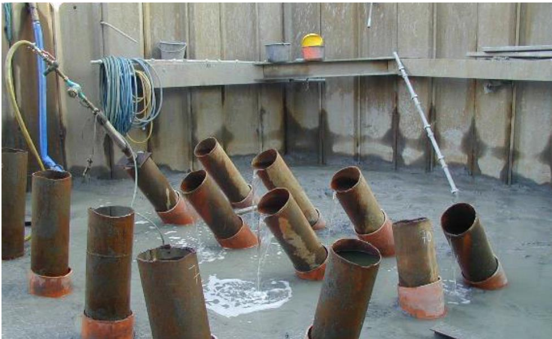
Figure 9: Seepage of ground water through open steel core pile casings.
