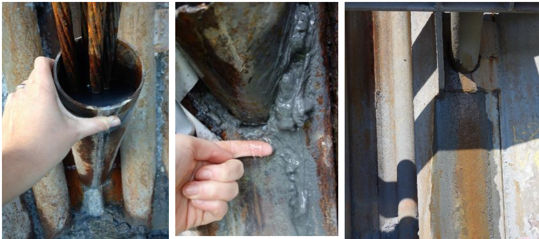
Figure 6 Example of leakage of water around and through casings for tie-back anchors.
