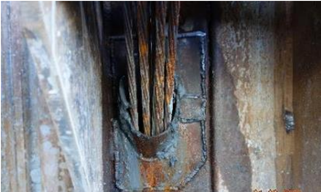
Figure 26: Steel plate welded onto sheet pile to cover hole opened during drilling of anchors (NGI).
