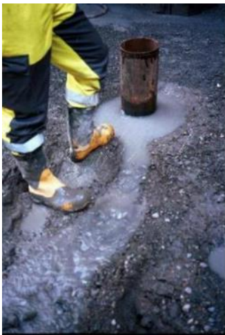
Figure 7 Example of leakage of water around casings for steel core pile at bottom of excavation (photo: Jernbaneverket).
