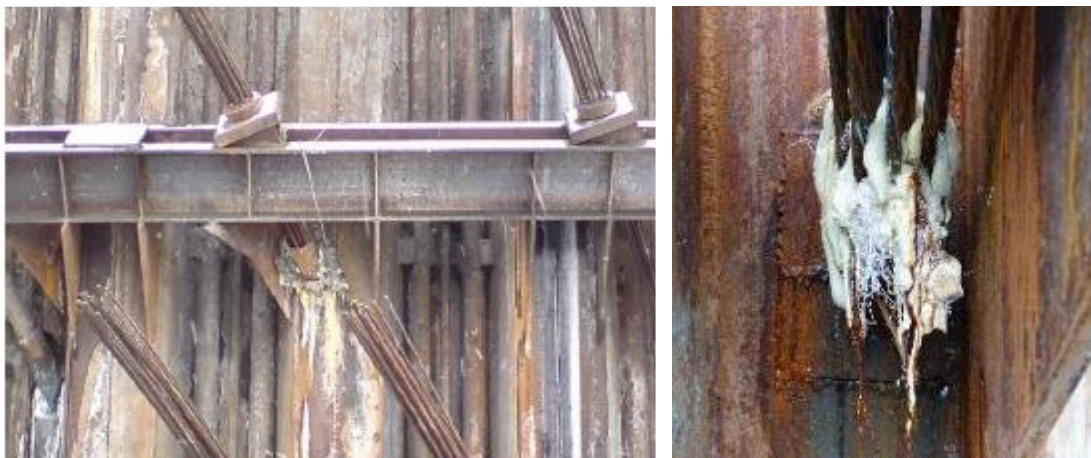
Figure 21: Left: Sealing of an opening for anchors with polyurethane grout (Picture: Huth & Wien Engineering AS). Right: Detail of opening for anchors after sealing (Picture: NGI)
