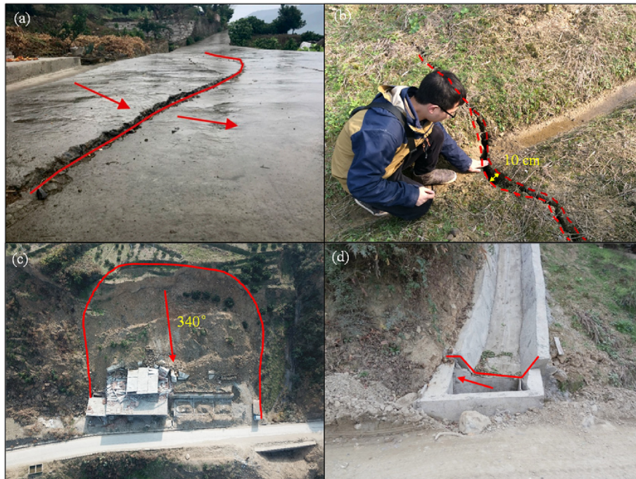
Fig. 4. Deformation on the Outang landslide: (a) Tension crack observed on the first sub-unit in 2017, (b) Crack observed on the east strong deformation zone in 2019, (c) Resident house and road destroyed by a local collapse in 2018, and (d) Destroyed drain on the second sub-unit in 2014 (Guo et al., 2020).
