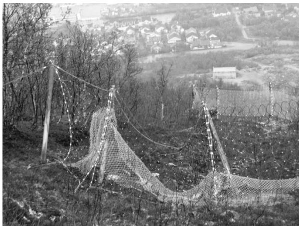
Figure 1. The photo shows an example of a structure in bad shape. These nets have now been replaced with steel bridges.
