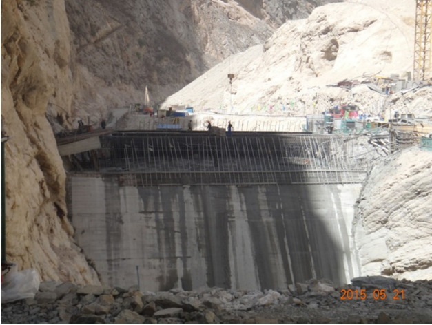
Fig. 2. The large concrete monolith across the river channel near completion - looking downstream (as described in the text, the monolith was constructed much larger than the optimum design required).
