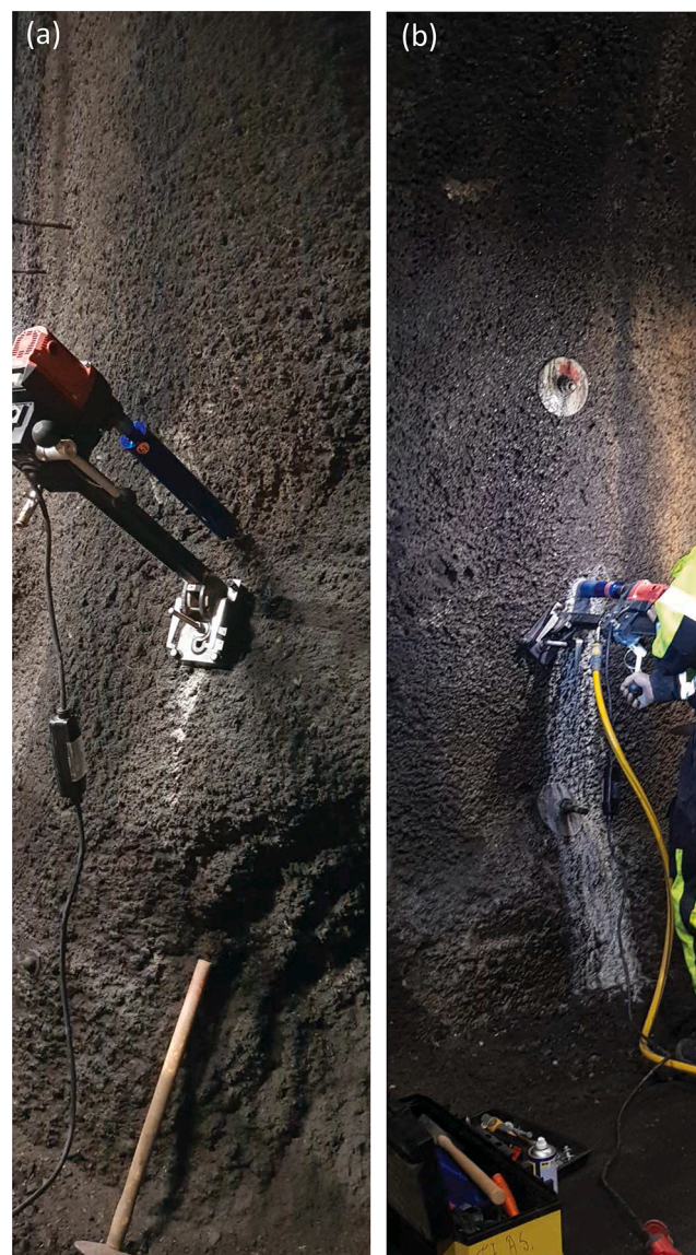
Fig. 5. Core drilling in: (a) Zone 1 located in the Nordkapp tunnel at chainage 3 + 220, and (b) zone 2 placed in the Nordkapp tunnel at chainage 4 + 920.
