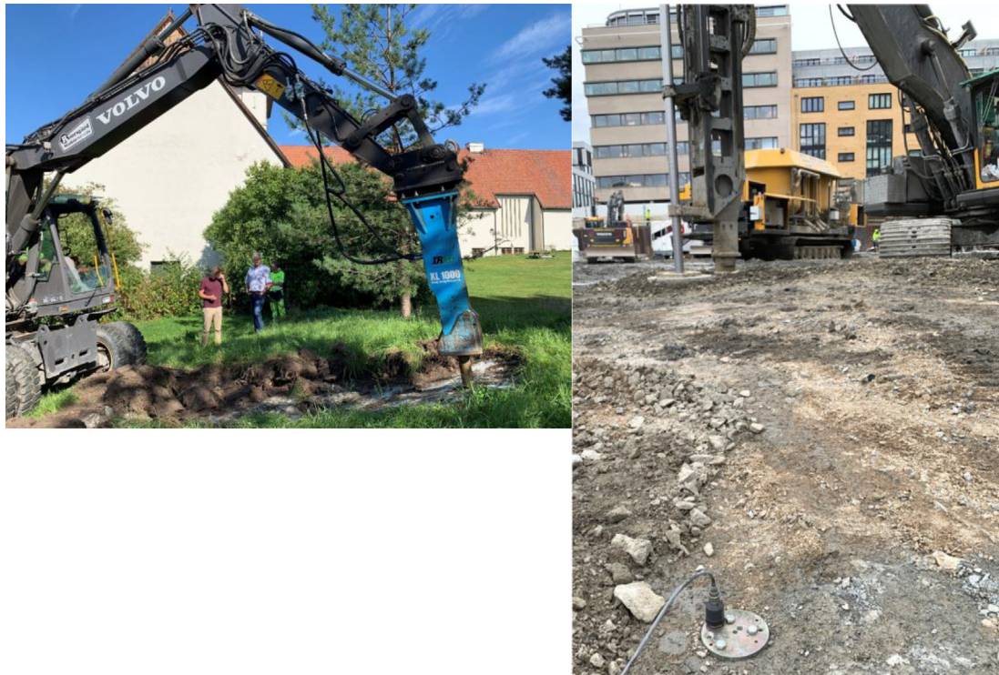
Fig. 9. Left: Excavator with hydraulic rock breaker tested at the museum site. To the left is the gable of the Gokstad wing and to the right the Oseberg wing. Right: Lime cement stabilization rig measured at site with similar ground conditions. The seismic accelerometer mounted on metal plate is seen in the front.
