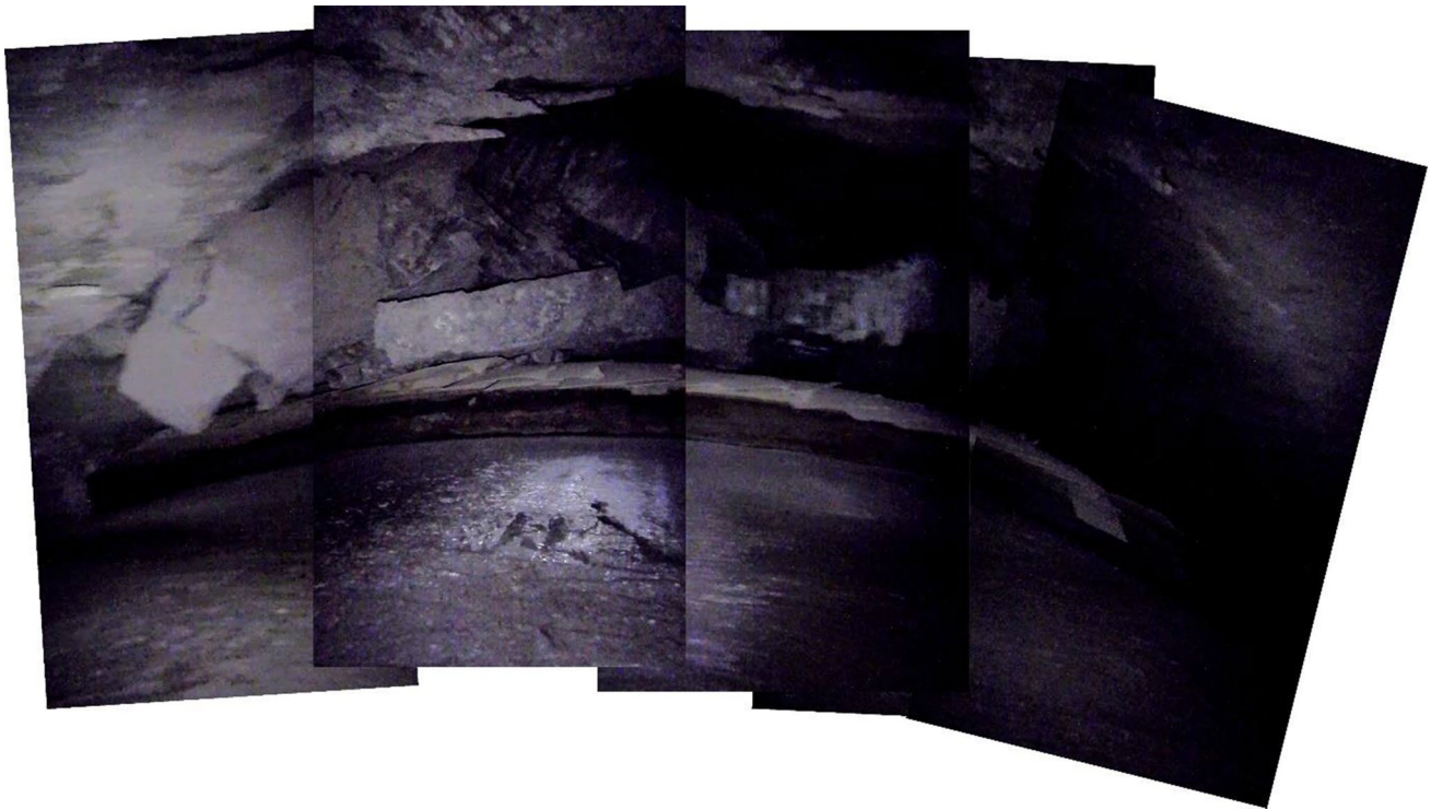
Fig. 4 Stitched panoramic view from a video recording out of an opening in precast concrete segments from behind a TBM-DS's shield. View direction is into advance direction. An overbreak caused up to m-sized blocks to be lying on the shield
