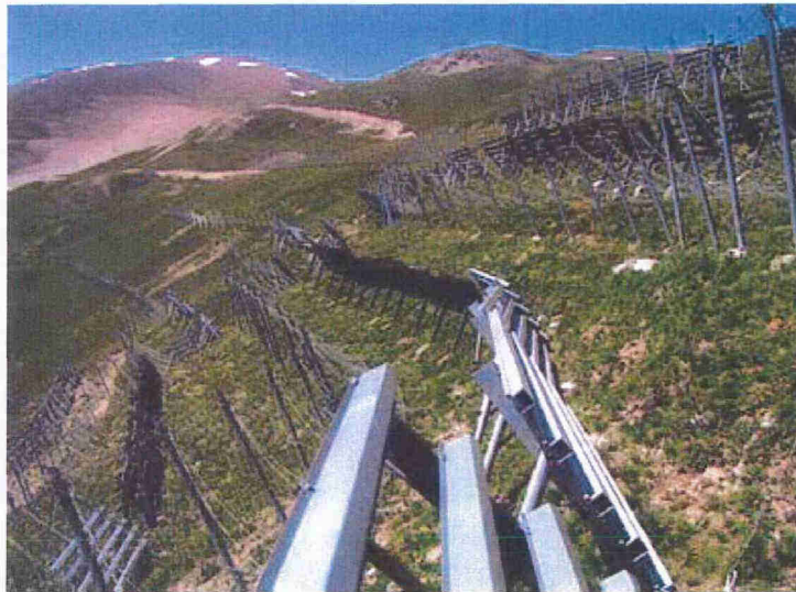
Figure 5.3 Side view of the release zone of the "Costraccia" avalanche, with the already existing rows of retaining defence works
