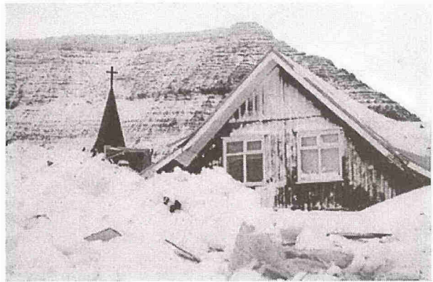
Figure 9. The 1 st floor of a house floated with the avalanche
