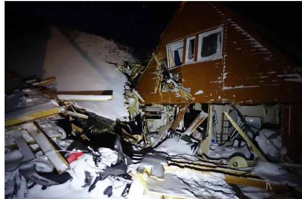
Figure 4: Example of massive damage. Photo: Kjetil Brattlien, NGI.
