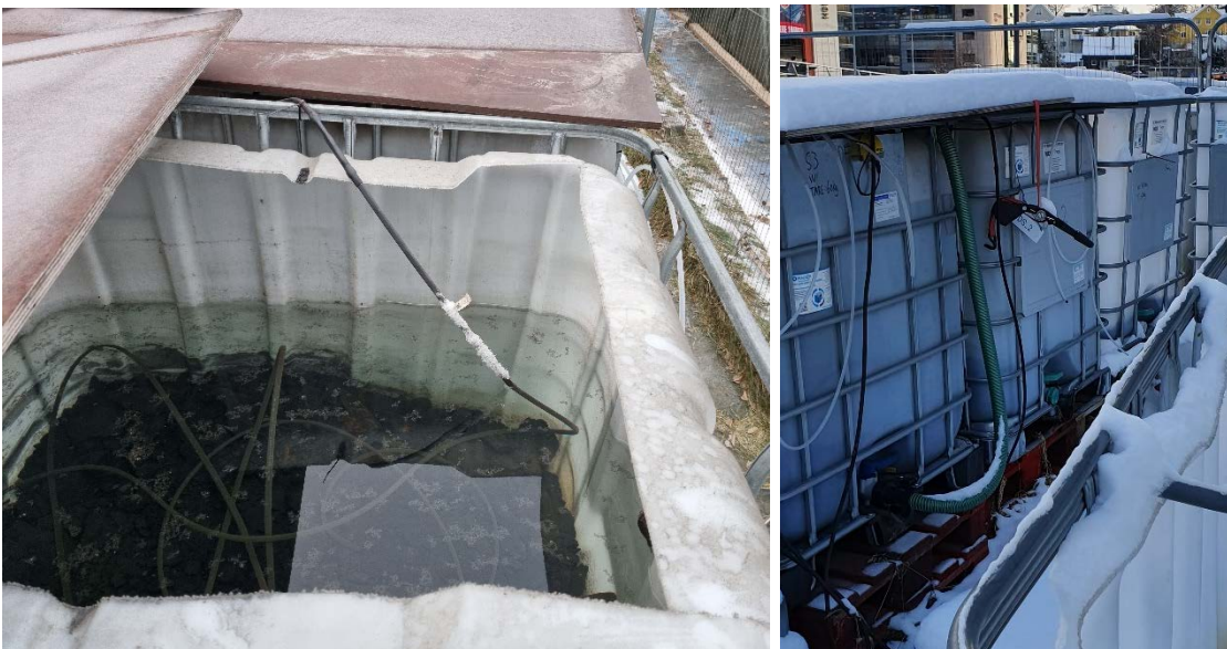
Figure 13 New lids of shuttering boards fastened with straps were installed to stop intrusion of rainwater. Left: looking down into one container (cable is for heating), 08.03.2022. Right: snow lying on top of lids, 02.02.2022.
