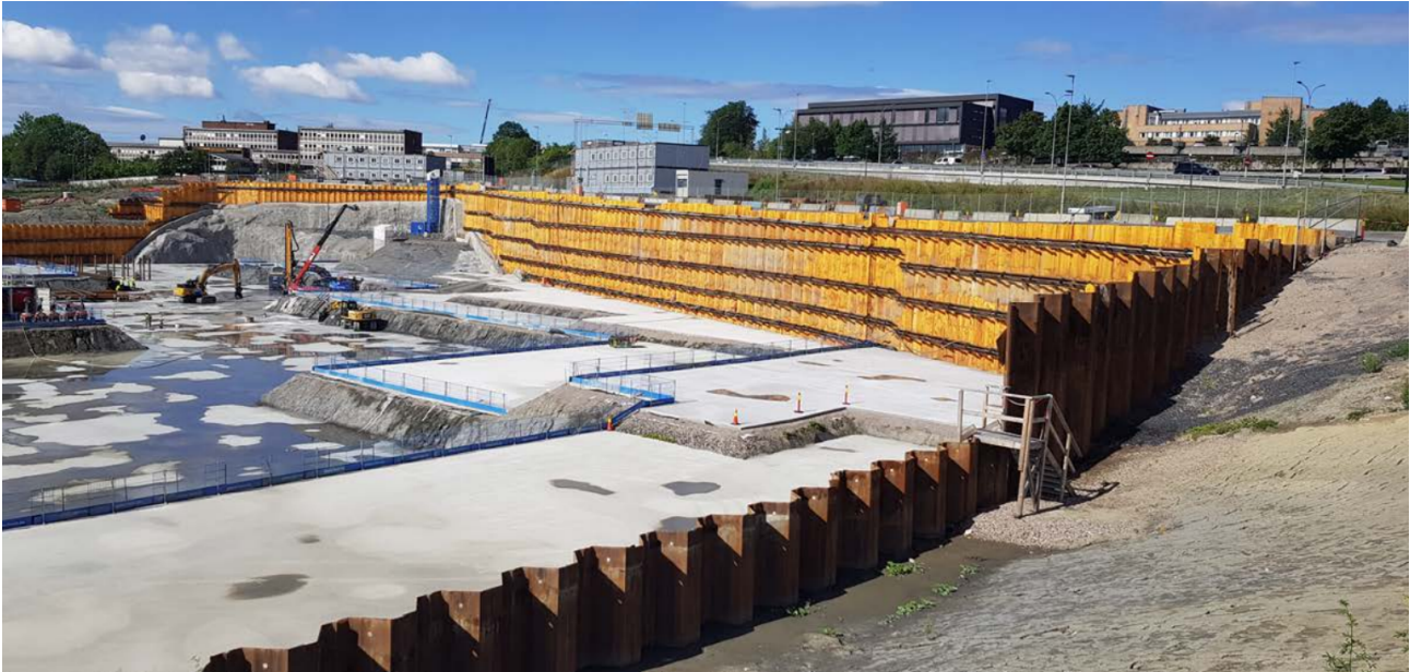
Figure 9: Construction site of the LVB with foundation, sheet pile walls and anchors [11]
