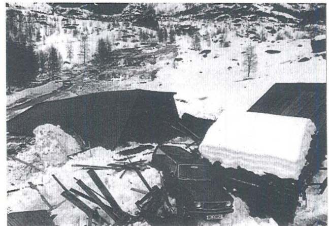
Fig. 4. A slushflow released at an elevation of 40 m above the farm destroyed four buildings. Average gradient of the path was 12.5°. Hjorteland, Suldal, West Norway, 3 March 1979. (Photograph by K. Strand, Haugesunds avis .)
