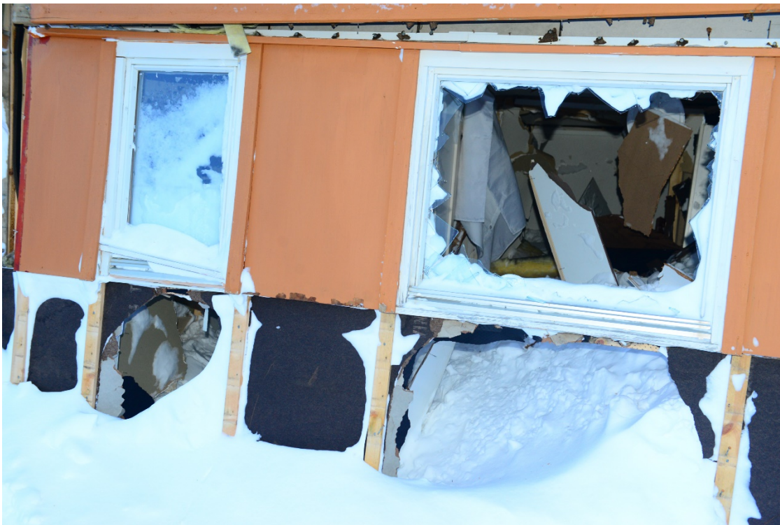
Figure 26 Avalanche in Longyearbyen, 2017-02-21: View of the damage area from above (top) and detail of the damage on the rotated house (bottom). Photo C. Jaedicke (NGI)
