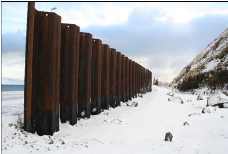
Figure 5 Sheet pile structure to stop rockfall and small avalanches. Photo A. Jonsson
