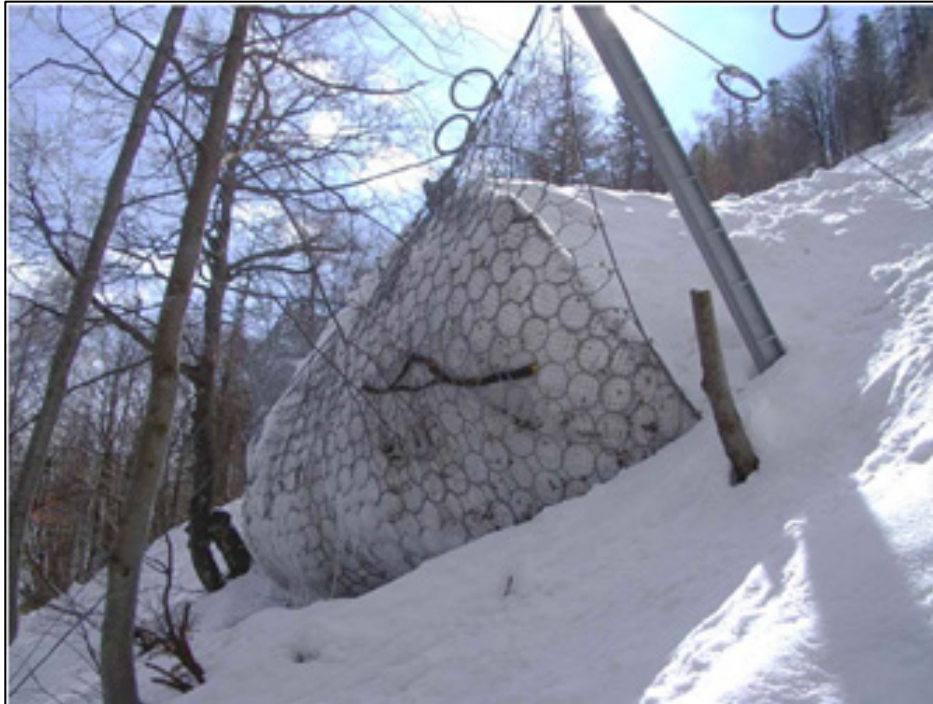
Figure 8 Barrier in Fieberbrunn, 15. April 2004 stopped a small avalanche (Photo Stefan Magreth).
