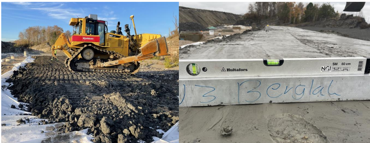
Figure 3. Compaction of the first of three layers (left). Sealing layer surface upon finalization (right).
