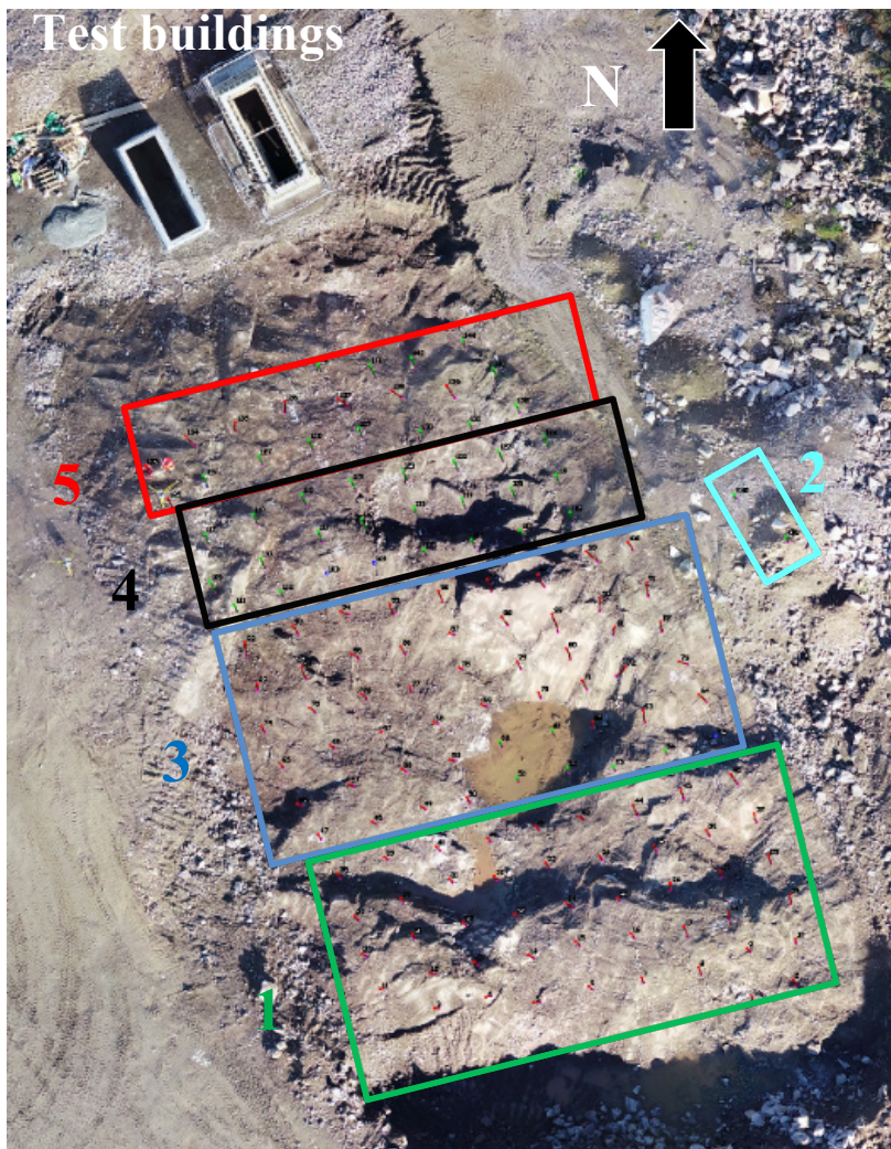
Figure 14. First blast test, localisation and numbering of the blast rounds. Test building in top left corner (Leca on the left and concrete on the right)
