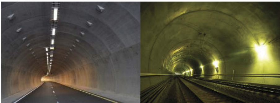
Figure 2. Photos of two completely drained lining systems from modern traffic tunnels. Left: The Nordic drip and freeze insulation lining system based on concrete segment structure. Courtesy Å. Homleid. Right: the conventional cast-in-place concrete lining system, Ulvin railroad tunnel, Norway.
